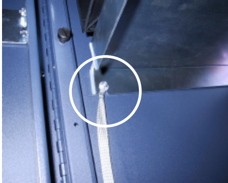
Figure 6. Grounding strap secured to dispenser tray mounting bolt.
