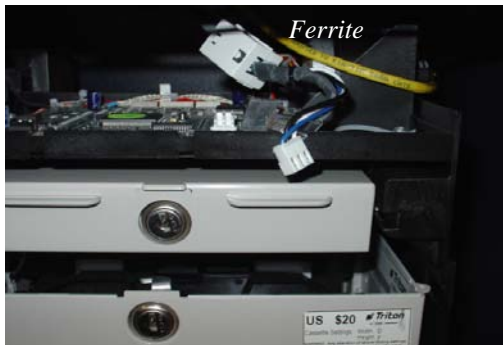
Figure 4. Power and Comm cable disconnected.
