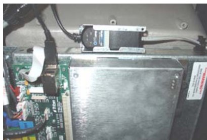
Figure 3. Modem secured and connected.
